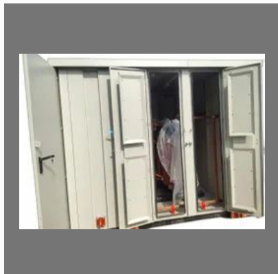
200 KVA Compact Substation
