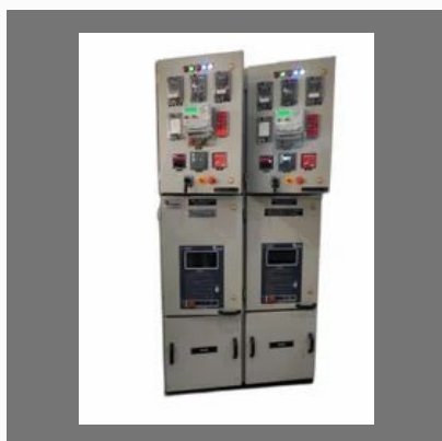
11kV VCB Panel
